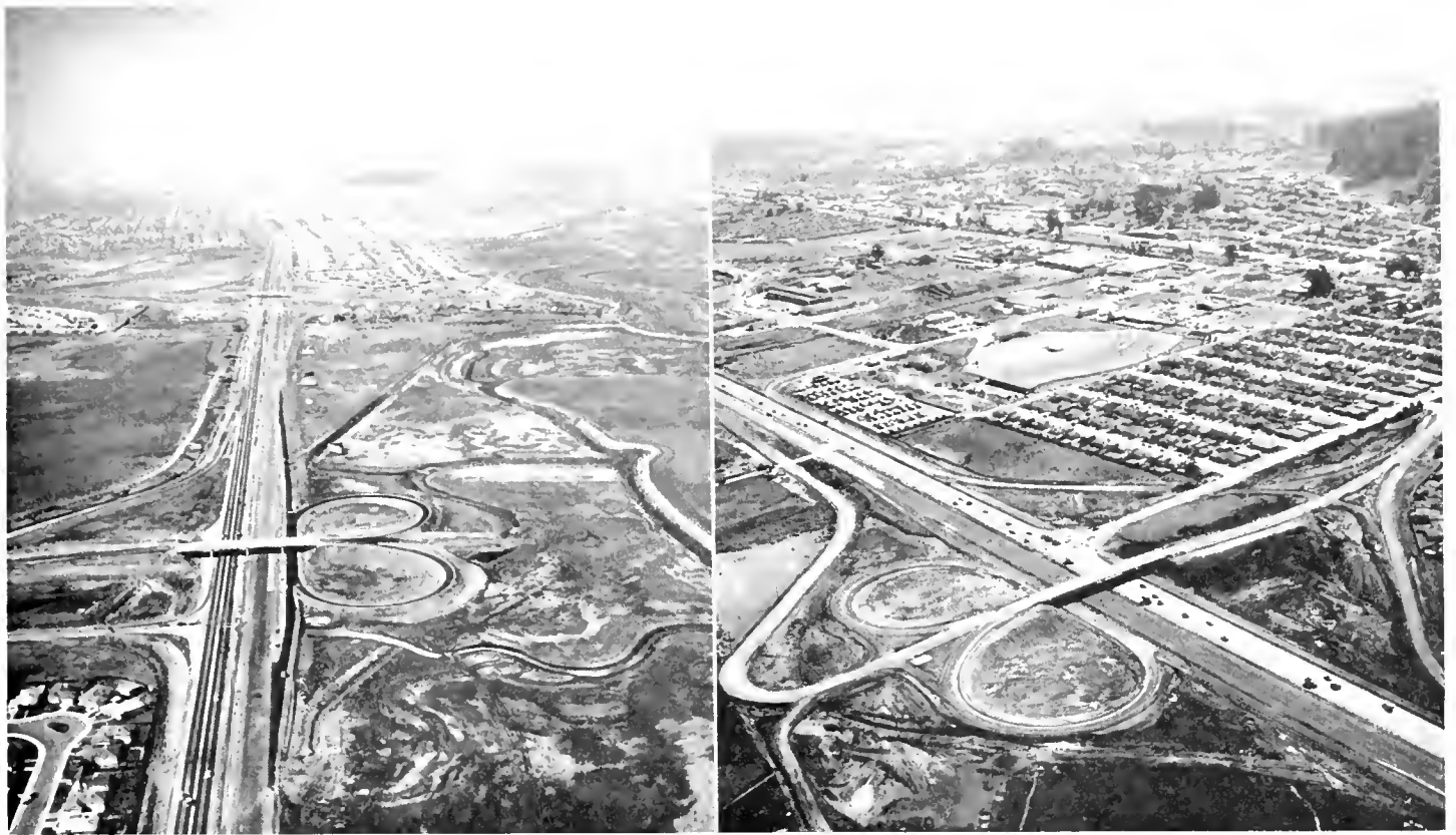
LEFT—View of Bayshore Freeway during final stages of construction looking north from vicinity of Hillsdale Boulevard interchange in San Mateo. RIGHT—View of Ralston Avenue interchange on Bayshore Freeway in Belmont near completion of construction.
